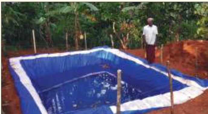
Inspection of water storage structure constructed at Rajakkad, Idukki under the scheme for Construction of Rainwater Harvesting Structure
